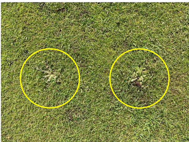
Figure 23: When voids appear in the grass cover, weeds, moss and undesirable coarse grasses are quick to invade.
